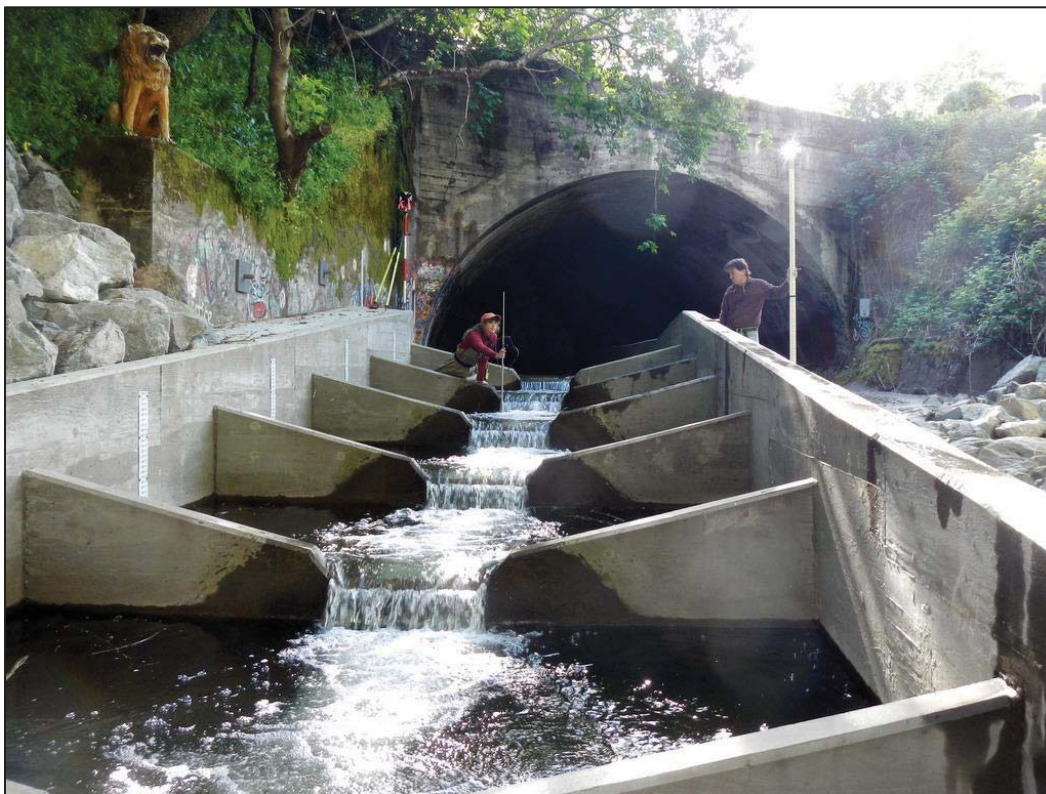
Figure 3. Downstream view of a partial-spanning pool-and-chute fishway in San Anselmo Creek, Marin County, California. 5
